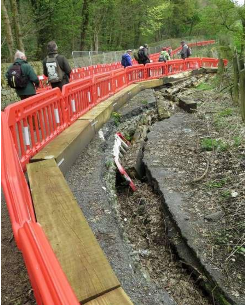
Landslip in the last year.
